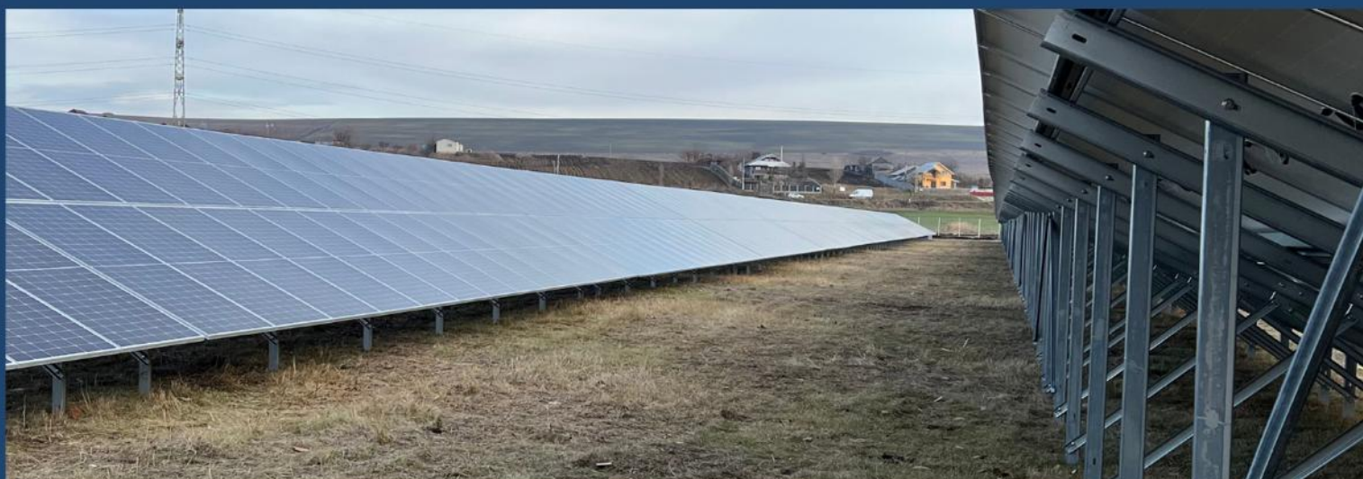
Premier Energy's CEF Frumuseni 0.5 MW solar park, near Arad, Romania
