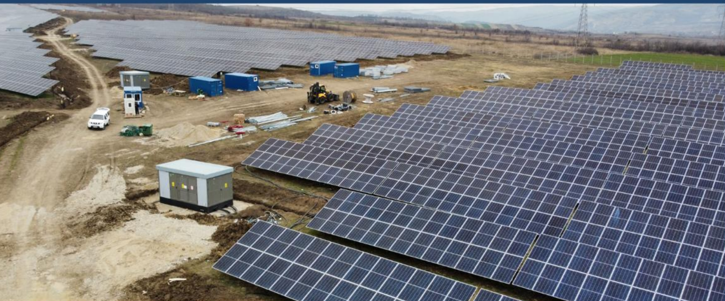
CEF Izvoru Barzii 14.8 MW solar park, Mehedinti County, Romania, managed by Premier Energy
