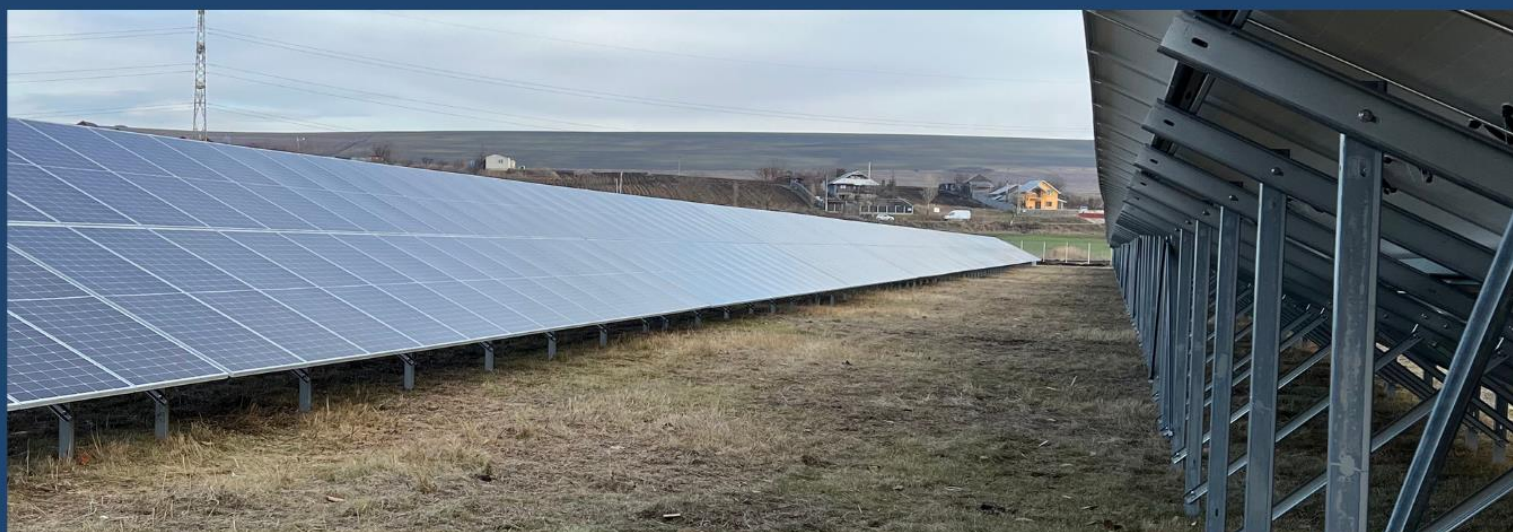
Premier Energy's CEF Frumuseeni 0.50 MWp Solar Park, near Arad, Romania
