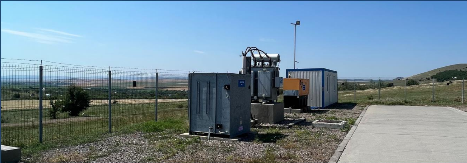
Premier Energy's ENEX 27.5 MW Wind/Solar Park station, Tulcea County, Romania
