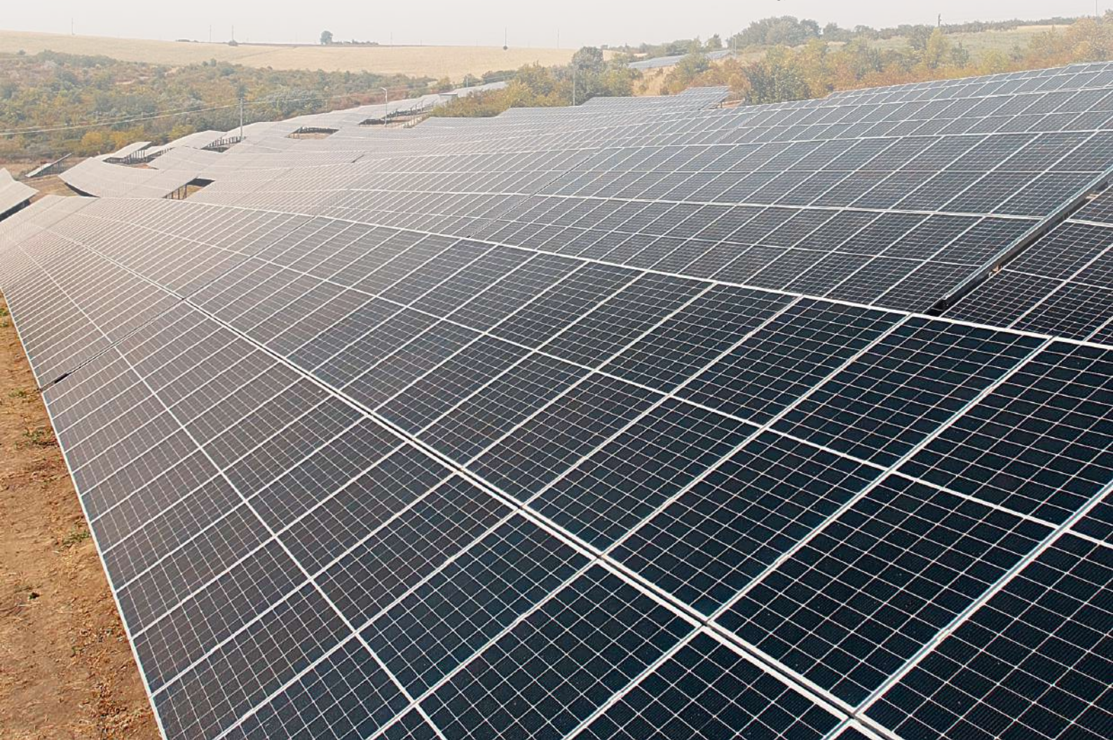
Premier Energy's Solar Park near Chisinau, Moldova
